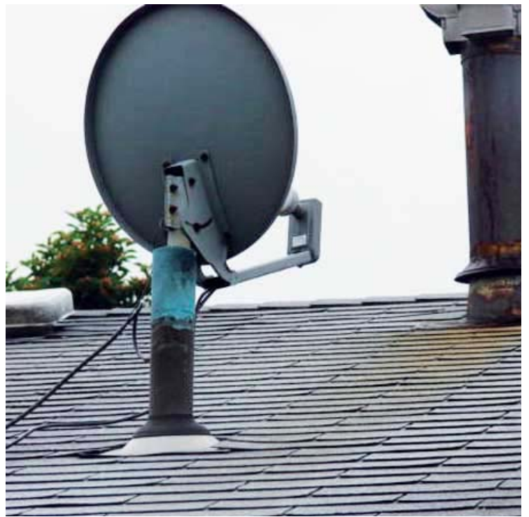
Can't mount it on the roof so let's use the vent stack.
