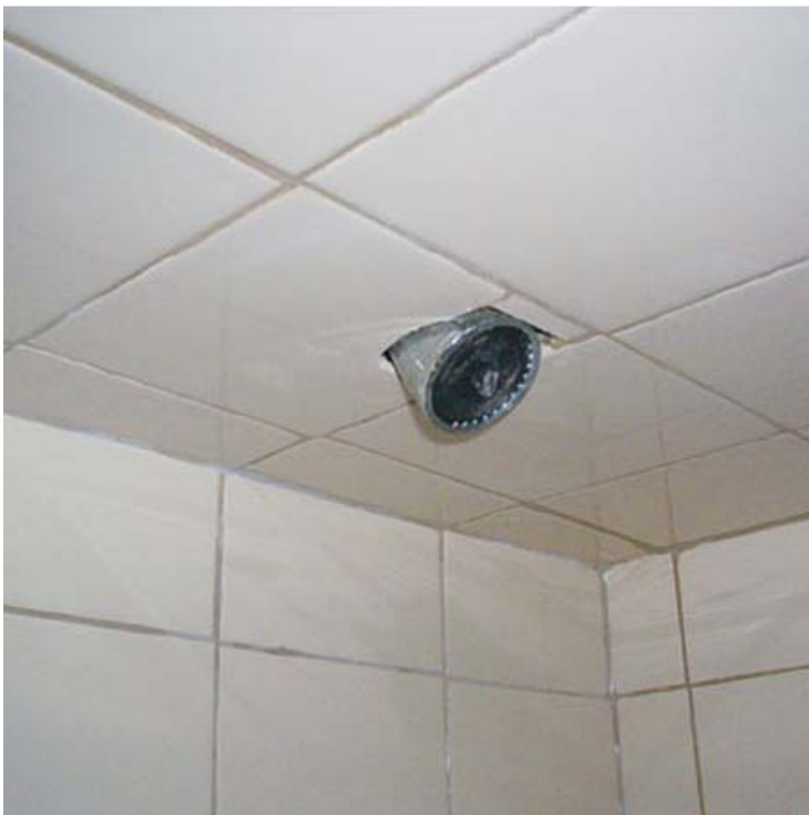
The ceiling was too low by a foot....
